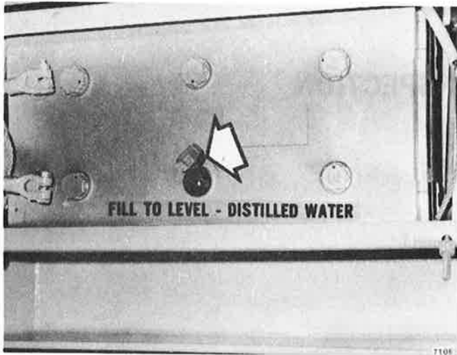
Figure 82 ELECTRICAL STORAGE BATTERY
