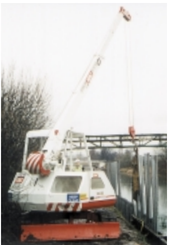
CX-3T Riverbank piling duties along narrow canal banks with site accessed under low bridges ▼
