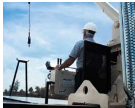
Boom trucks and truck-mounted cranes
