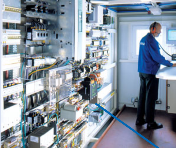
Air-conditioned electrics compartment
