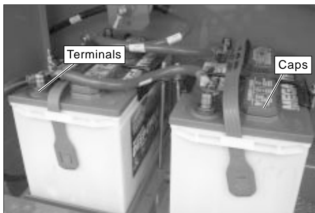
Figure 7.6 – Emergency Power Battery
