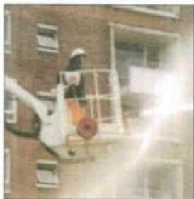
Water jet and fog curtain.
